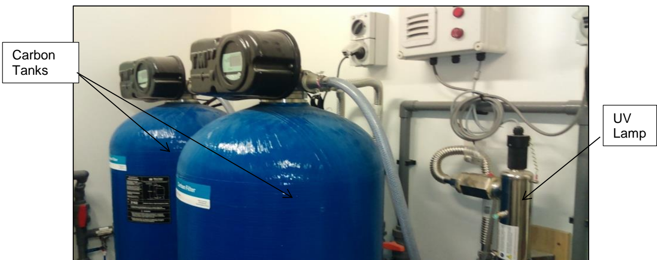
(Plant Room Tamworth Dialysis Unit HNE Health)
