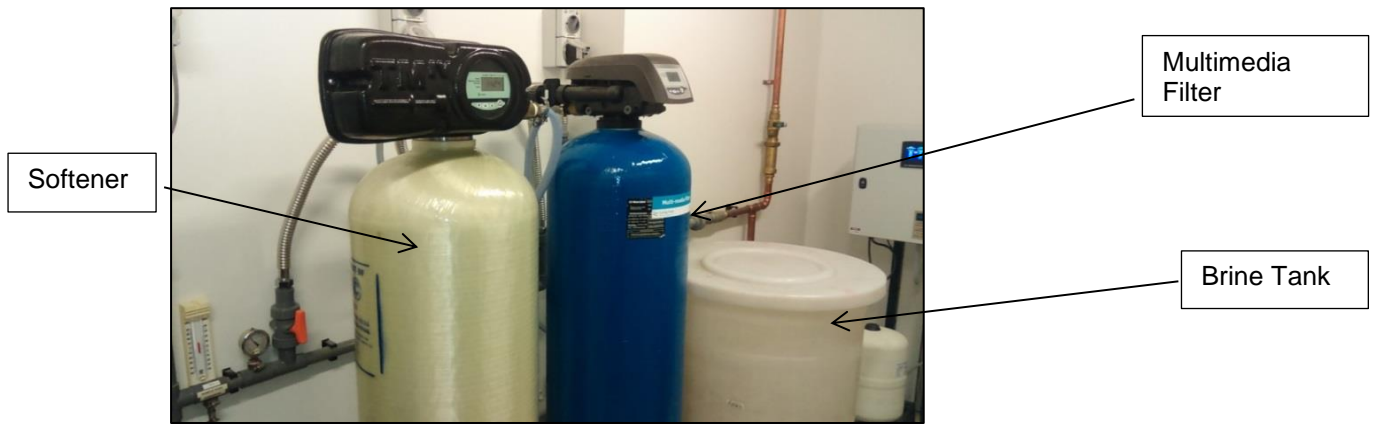
(Plant Room Tamworth Dialysis Unit HNE Health)
